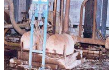
Pumps in wet atmosphere
