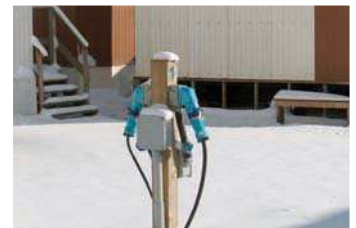
External power supply for water treatment
