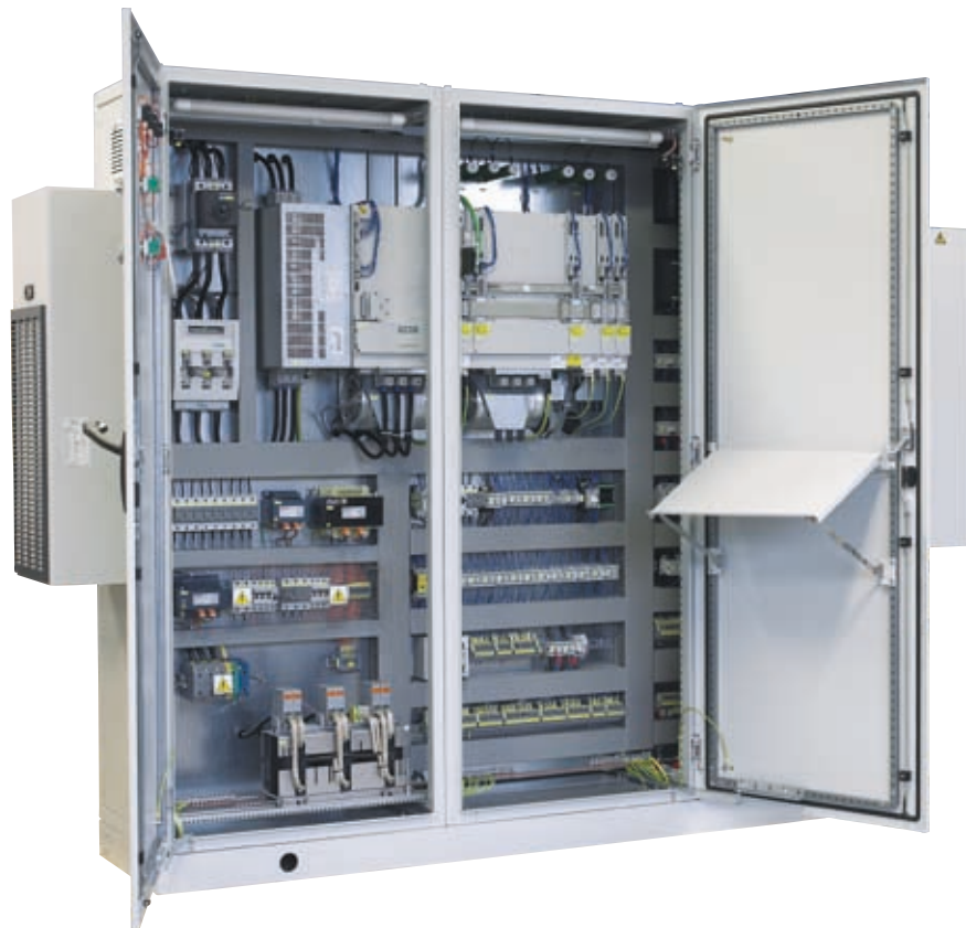
Control cabinet for Machine Tool Factory RAFAMET S.A.
