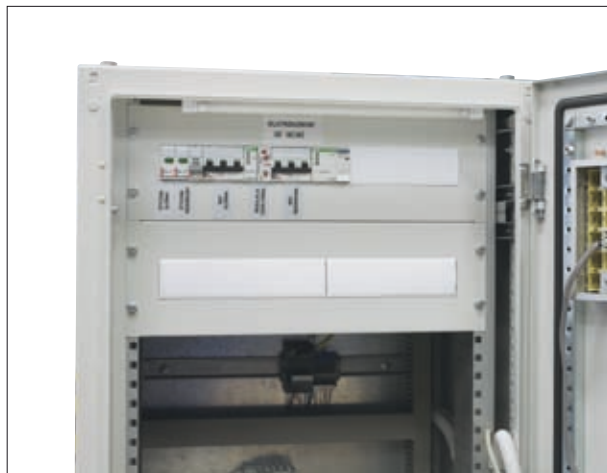
Relay-based ATS system mounted in a cabinet
