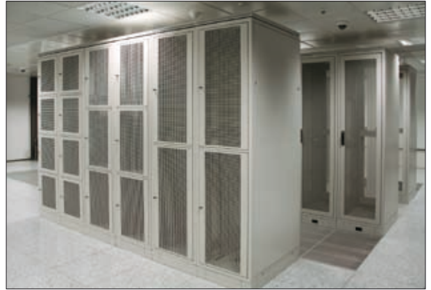
SZB DC cabinets installed in the server room of ATM S.A. in Warsaw
