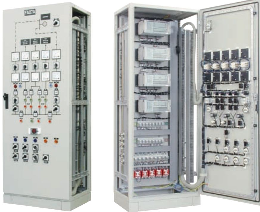
ATS system for multiple incoming feeds, based on the control panels of Energotest-Energopomiar, made for the Wielopole power station
