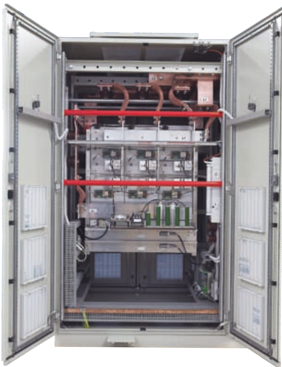
Excitation cabinet for 600 MW generator - rectifier box
