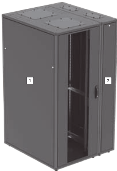
1 - server cabinet, 2 - management cabinet
