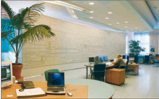
Regional Power Dispatch Facility in Ostrołęka
