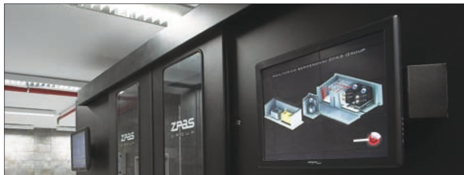
Example of server room monitoring visualization
