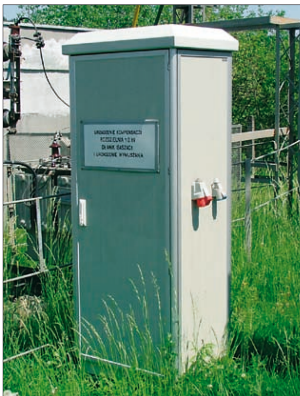
Cabinet for electrical substation earthing
