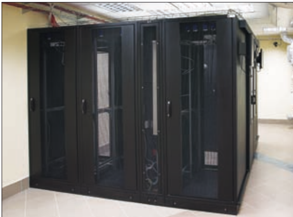
ZPAS Data Box installed in Gorzów CHP Station
