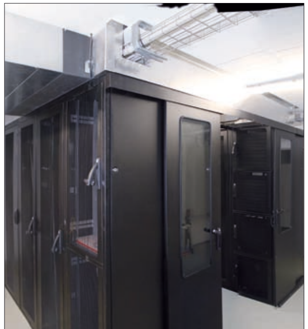
ZPAS Data Box installed in eM-I.T. in Bad Ischl, Austria
