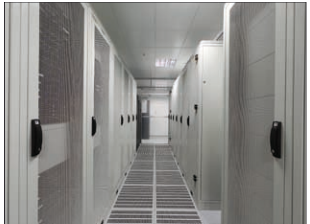
SZB DC cabinets installed in the server room of ATM S.A. in Warsaw
