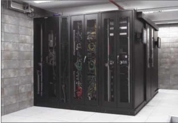
Data Box in the server room of ZPAS S.A. facility in Przygórze
