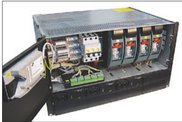
MPSU Flatpack2 power unit
